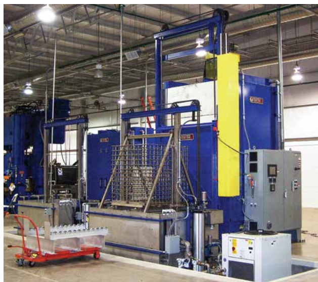
Fig. 6. Horizontal quench system located in a pit (courtesy of Wisconsin Oven Corp.)
